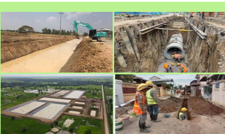
Exhibit 16: Main canal rehabilitation; drainage and sewage system construction; wastewater treatment plant construction; connecting sewage system to household. (Clockwise from top-left) © Battambang Provincial Hall
